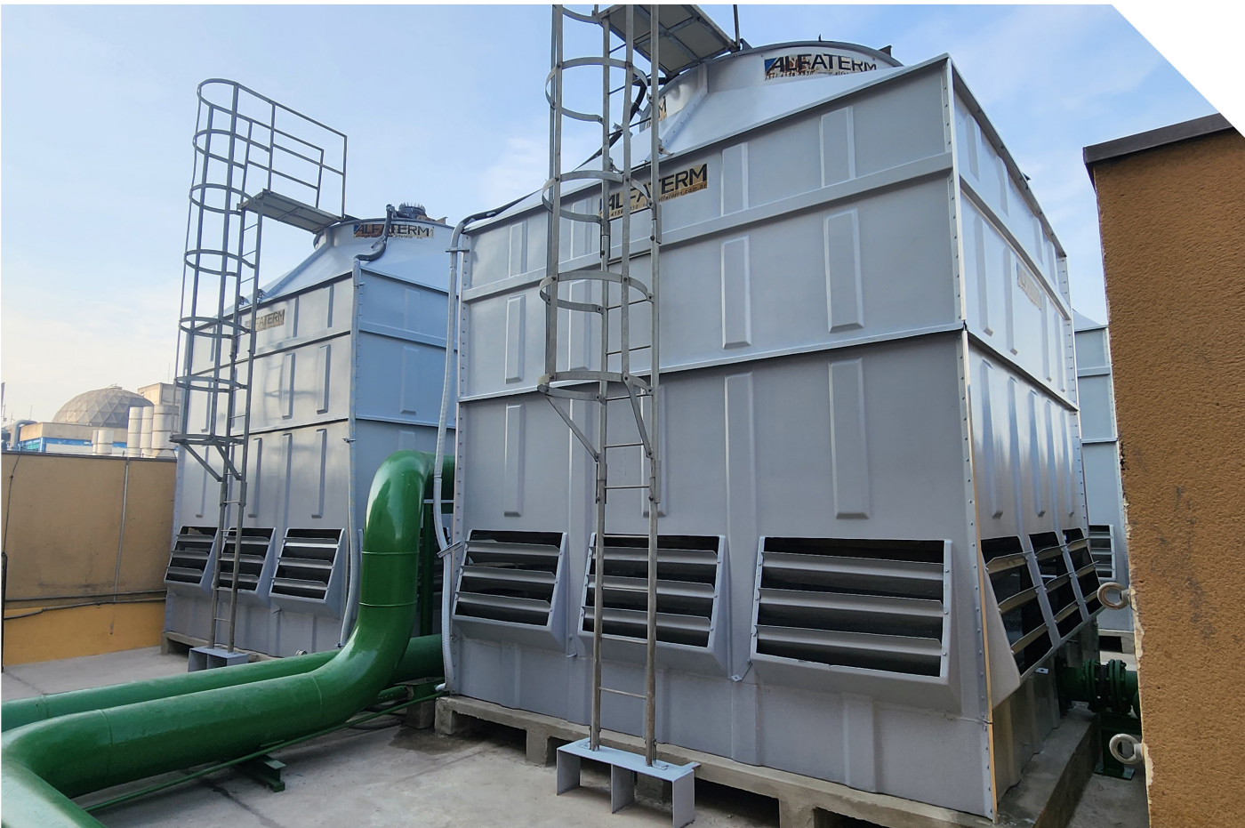
THE INSTITUTE'S COOLING TOWERS
